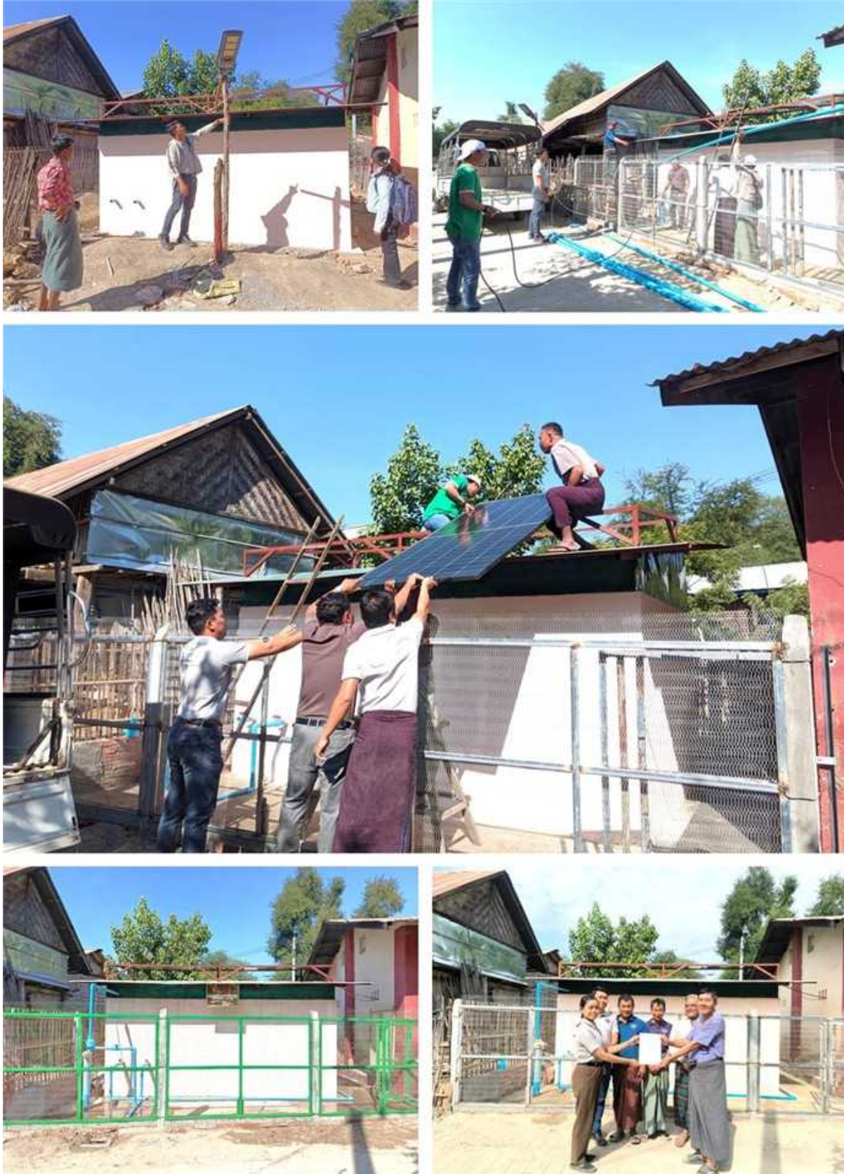
Figure 76: Completing Water Well Drilling, Concrete Water Tank Construction, and Solar-Powered Water Pumping System Installation at Chin Taung Village
