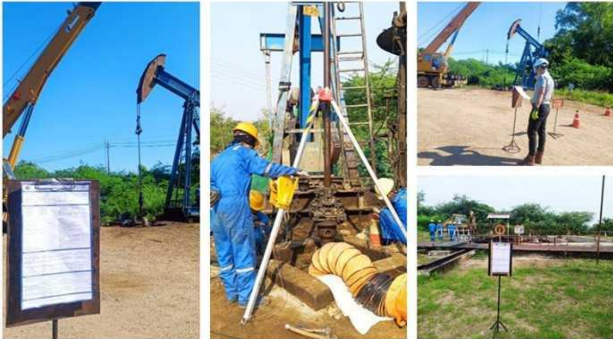
Figure 53: Permit to Work (PTW) Audit
