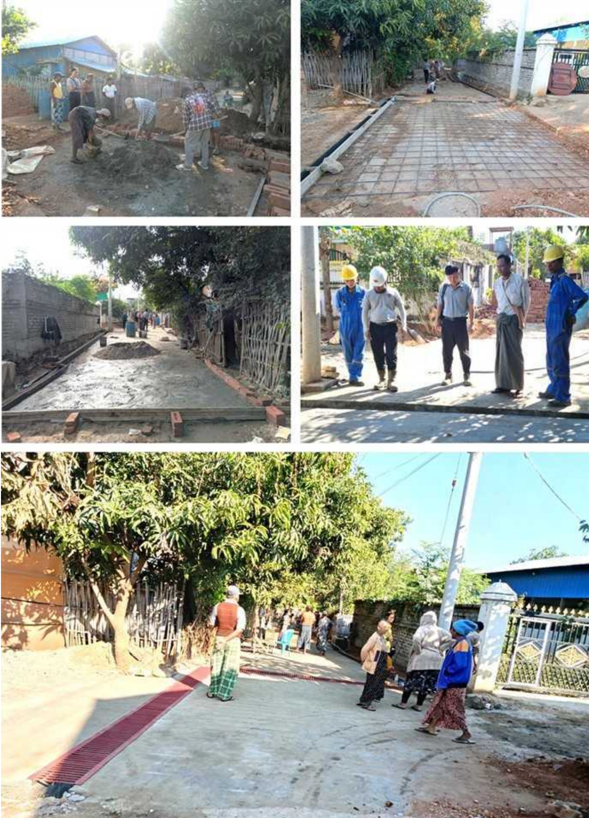
Figure 73: Completing Concrete Approach Road Construction and Drainage System in Aye Mya Village
