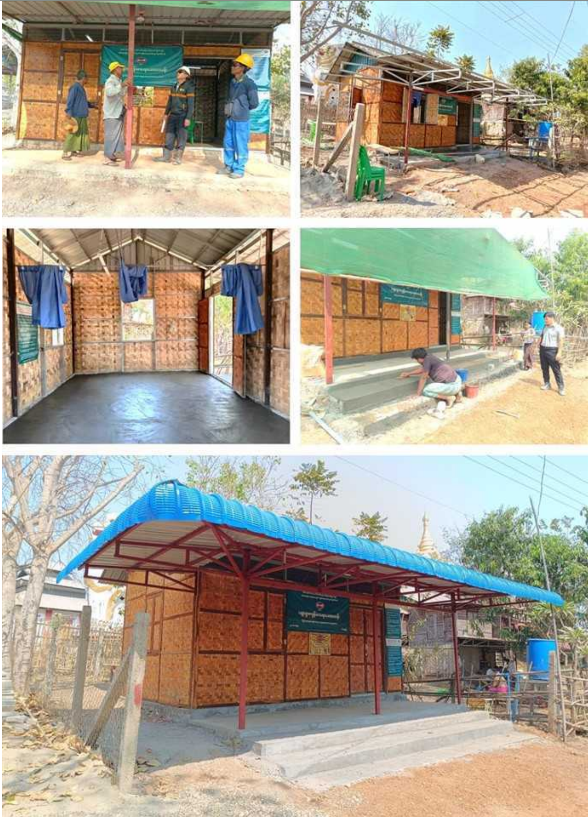
Figure 79: Completing Concrete Flooring and Sunshade Installation at the Former Library Site in Ywar Thar Village
