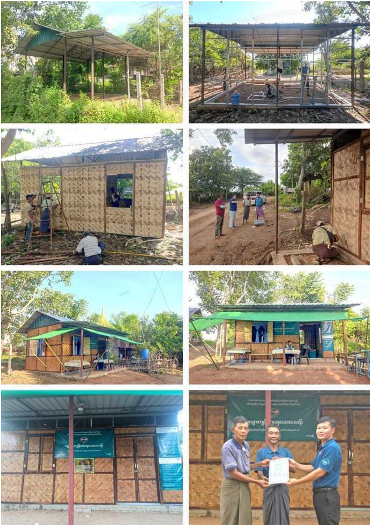
Figure 67: Completing the Construction of a Bamboo-Woven Structure at the Former Library Site in Ywar Thar Village
