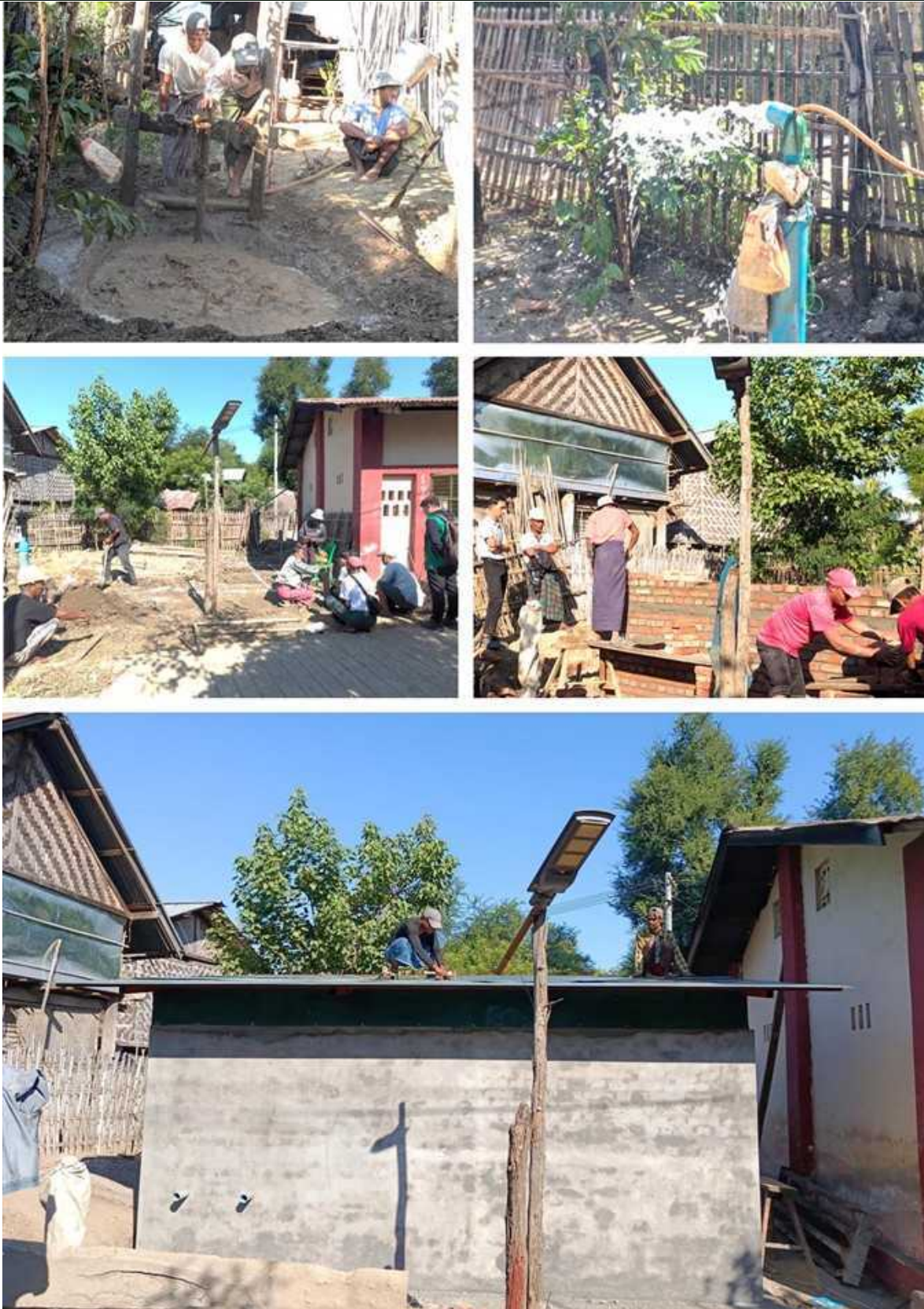
Figure 75: Monitoring Water Well Drilling, Concrete Water Tank Construction and Solar-Powered Water Pumping System in Chin Taung Village
