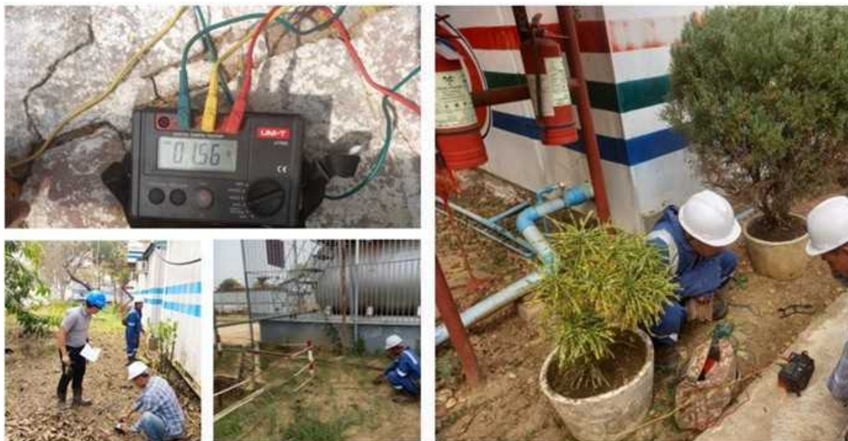
Figure 61: Earthing Resistance Test
