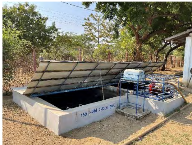
Figure 41: Warehouse Zero Discharge Tank
