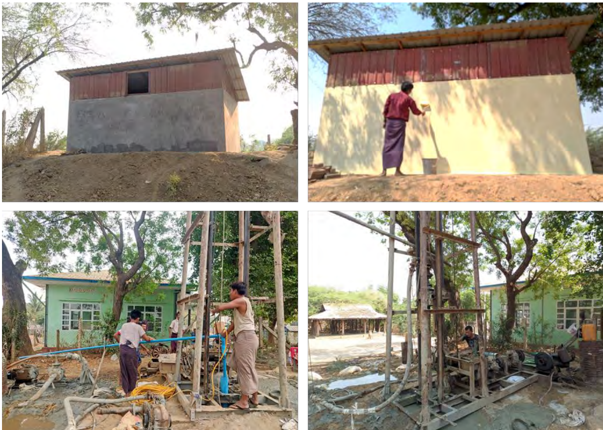
Figure 73: Monitoring the Progress of Concrete Water Tank Construction and Water Well Drilling at Kyar Kan Village
