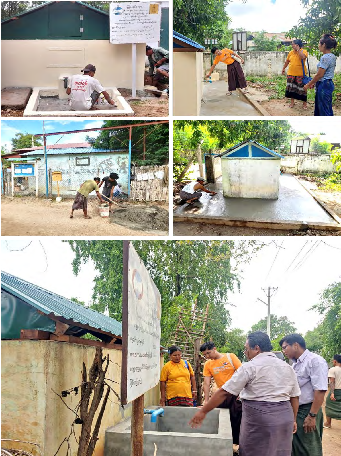
Figure 95: Renovating Old Water Collection Tanks at Kyar Kan, Mei Bayt Kone, and Auk Kyaung Villages
