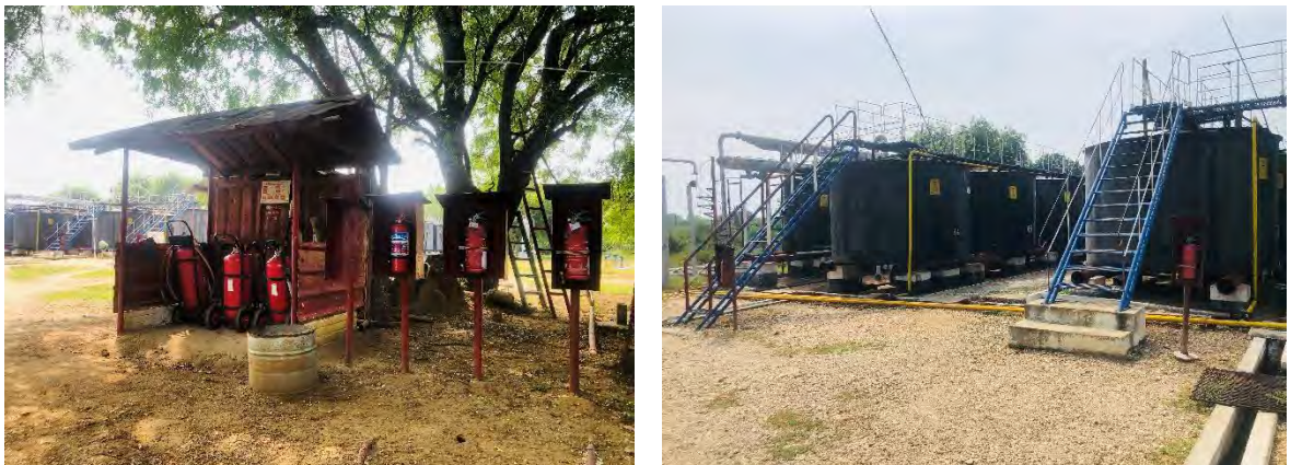
Figure 26: Fire Extinguishers at GOCS-2 and GOCS-3
