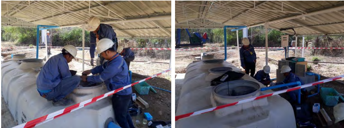
Figure 47: Desludging and Third-party Regular Maintenance of Bio-filter
